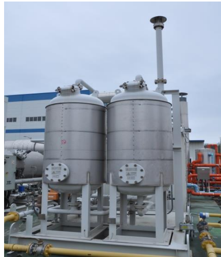
Desulfurization for Molten Carbonate fuel Cell
